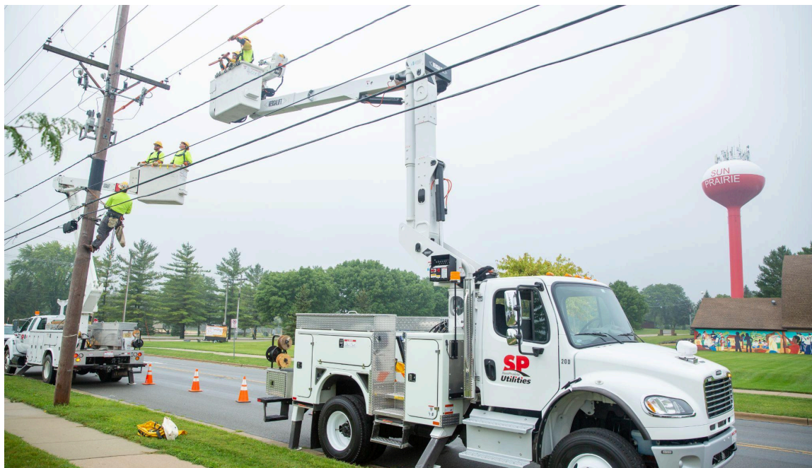
(2022 Photo: Sun Prairie Utilities lineworkers working on S. Bird St. in Sun Prairie.)
